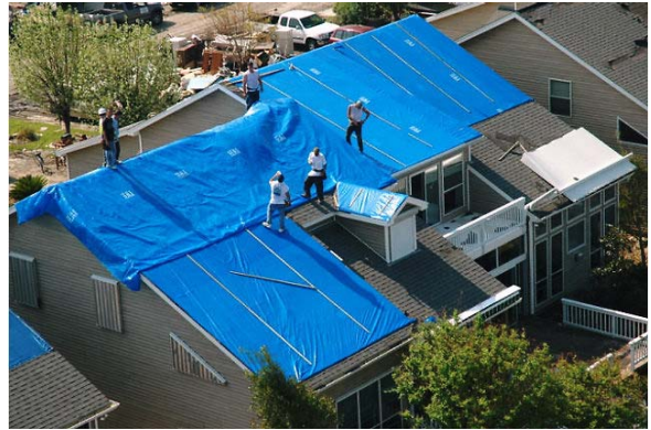
Shaw repairs tens of thousands of roofs in Louisiana in response to Hurricane Katrina.
