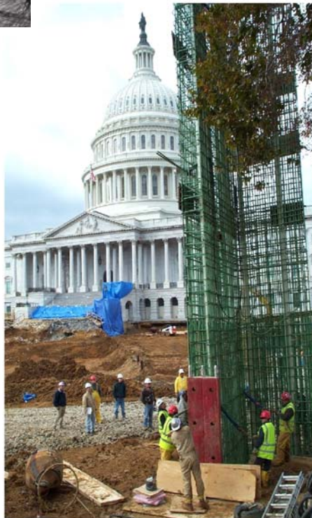
US Capitol Visitors Center, Washington DC - ECS is currently operating an on-site laboratory and is providing all testing and inspection services during construction for this new underground project. ECS is also performing geotechnical drilling services as part of the caisson foundation construction.
